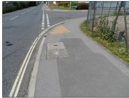
PHOTOGRAPH 5 EXISTING VODAFONE CHAMBER ON BRUNEL ROAD AT JUNCTION WITH EXETER WAY TO WEST OF SITE
