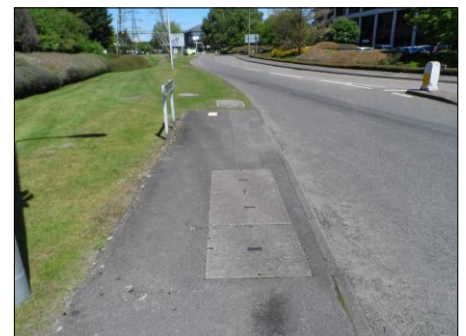
PHOTOGRAPH 3 EXISTING BT AND VIRGIN MEDIA CHAMBERS IN FOOTWAY / VERGE ON WEST SIDE OF WATERSIDE DRIVE
