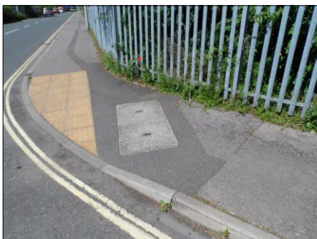
PHOTOGRAPH 1 EXISTING BT CHAMBER IN FOOTWAY ON BRUNEL ROAD TO WEST SIDE OF ENTRANCE (SERVING CHAMBER)
